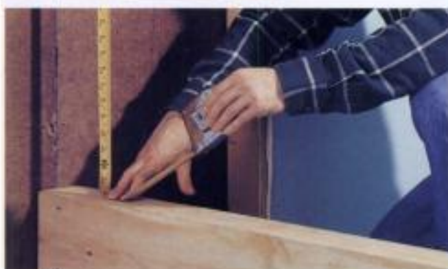
Removing interior load-bearing walls is covered on pages 188 to 191. Make sure to create temporary supports (pages 182-185) before removing or altering load-bearing walls.
