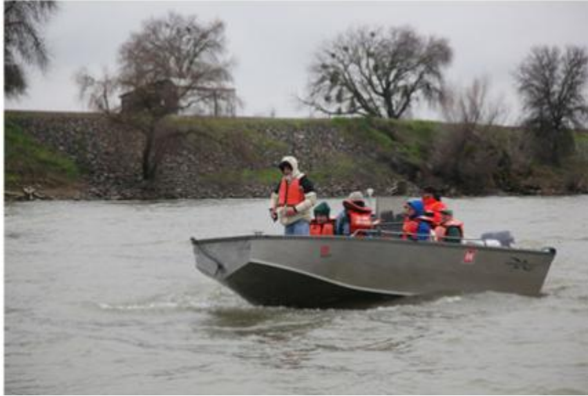
Figure 2 - Levee inspection by boat (Source: U.S. Army Corps of Engineers Digital Visual Library, 2010)
